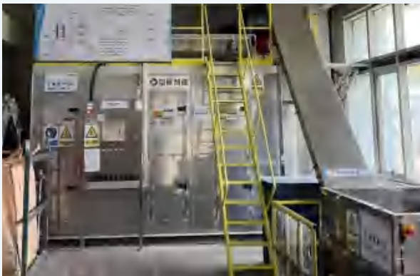
Wastewater treatment equipment
