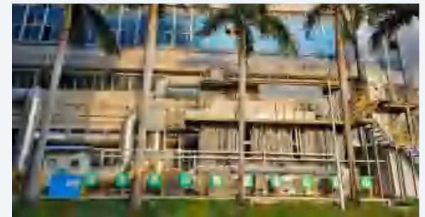
Waste gas treatment equipment
