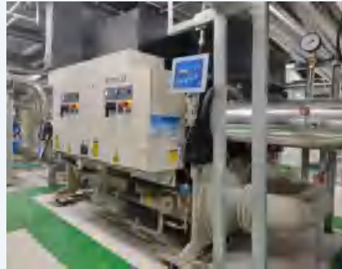
Air conditioning unit in Shenzhen Metro
