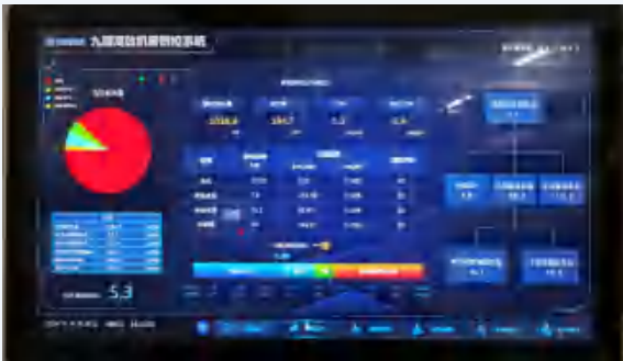
Improving energy efficiency in the air conditioning machine room of Zhuhai headquarters
